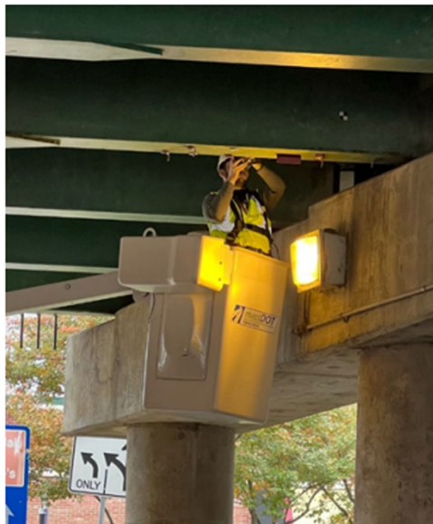
Fig. 4 | Inspection and structural integrity evaluation of an in-service bridge. Field-based 3D scanning with portable equipment. Replicated from Tzortzinis et al. 9
